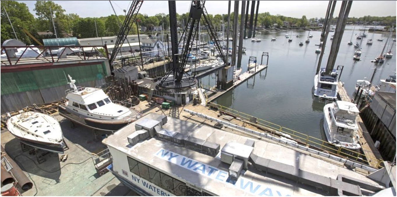
Figure 88: A ferry used in New York City being repaired at a boatyard located on the Harbor (photo by Derektor Shipyard)
