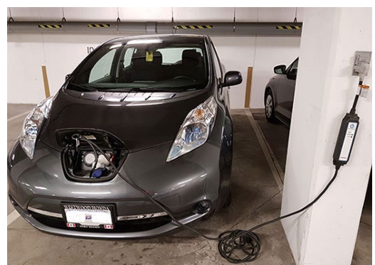
Figure 164: An electric vehicle is being recharged inside the parking structure of an apartment building.
