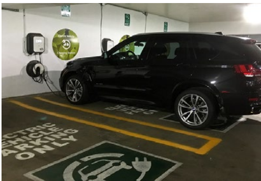
Figure 55: A parking garage retrofitted to include space for electric vehicle charging stations (photo by flickr user Mario Duran-Ortiz, licensed under CC BY SA 2.0)
