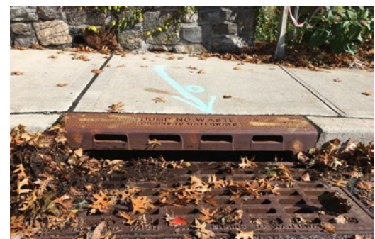
Figure 153: A newly-installed catch basin in the Village.
